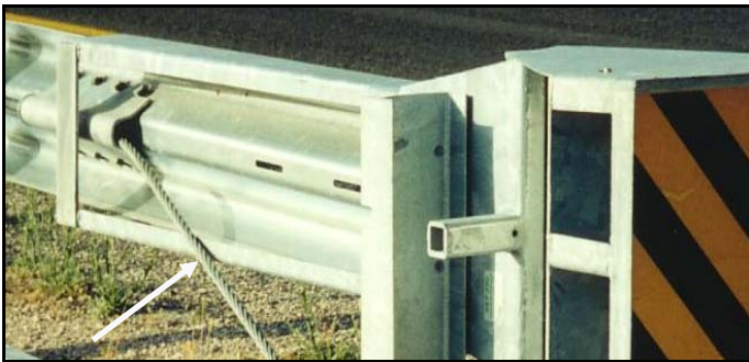
The SKT-SP cable is fed inside through the feeder chute. The SKT feeder chute is longer than the FLEAT
