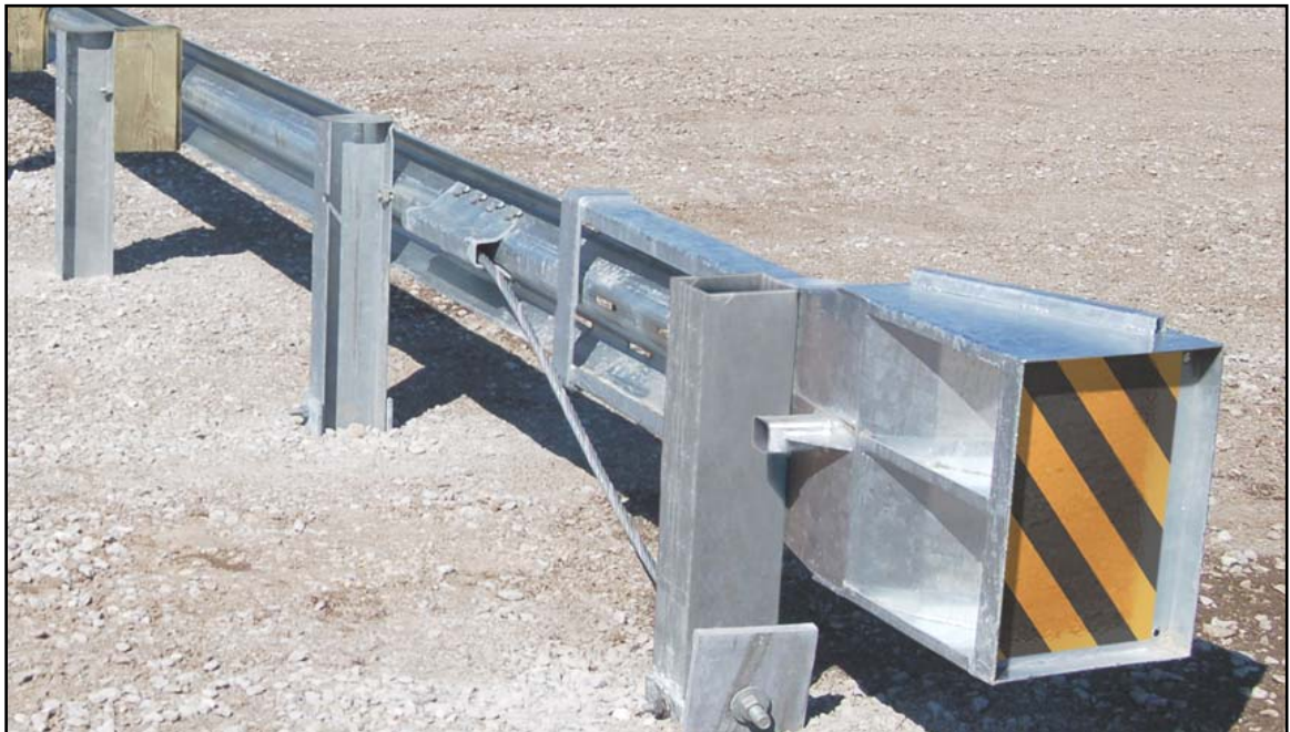
Figure 5. View of FLEAT-SP Steel End Post #1
