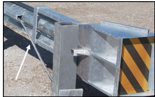
The FLEAT-SP cable NOT to be fed inside the feeder chute
